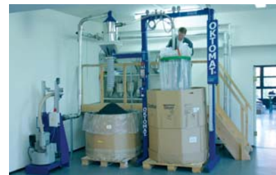
Refilling station with vacuum station
