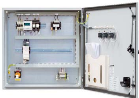
Internal View of 1 Fan Dry Cooler Stage Control Panel
