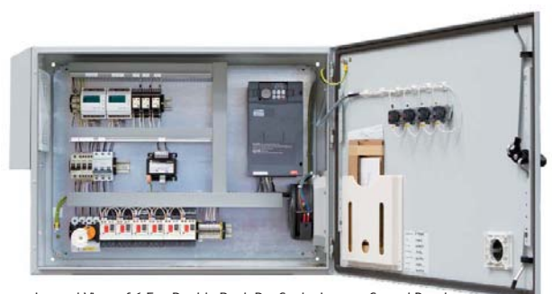
Internal View of 6 Fan Double Bank Dry Cooler Inverter Control Panel
