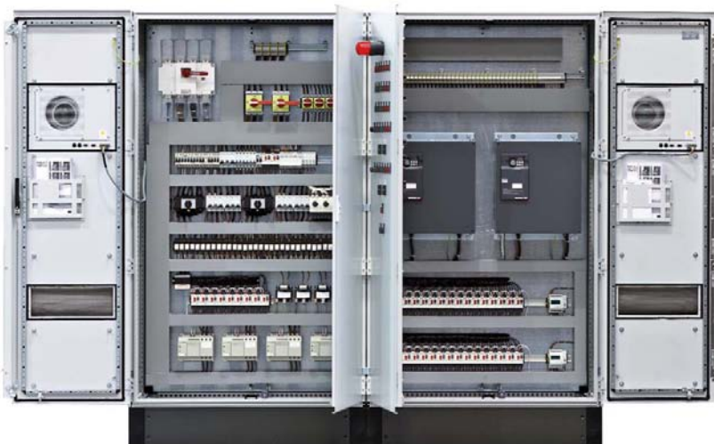
Internal View of Special 2 x 14 Fan Inverter Controls with the Addition of Multiple Status Lamp Indication, 2 x 15kW and 2 x 18kW Soft Start Run and Standby Pump Control
