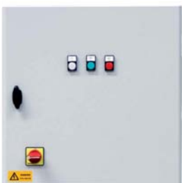
1 Fan Dry Cooler Stage Control Panel
