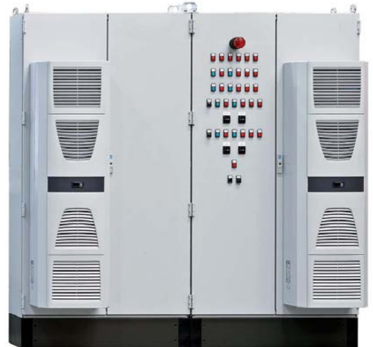
Special 2 x 14 Fan Inverter Control Panel with the Addition of Multiple Status Lamp Indication, 2 x 15kW and 2 x 18kW Soft Start Run and Standby Pump Control (1)
